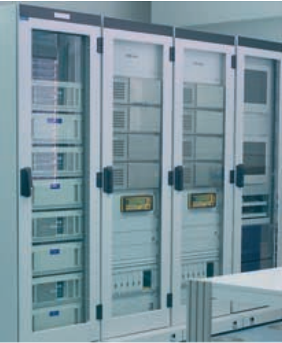
FIG 8 Central Switching Control Node DMX-600
