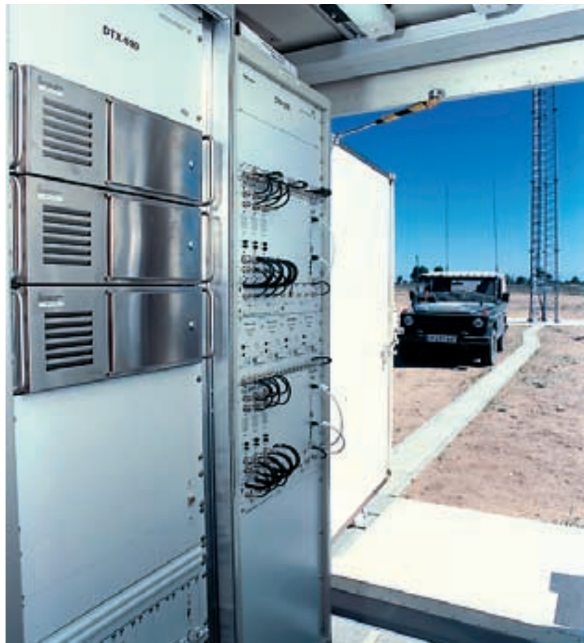
FIG 7 TETRA Base Station DTX-500
